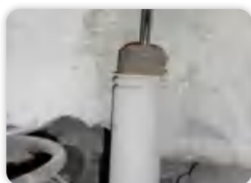
Loose bump stop
